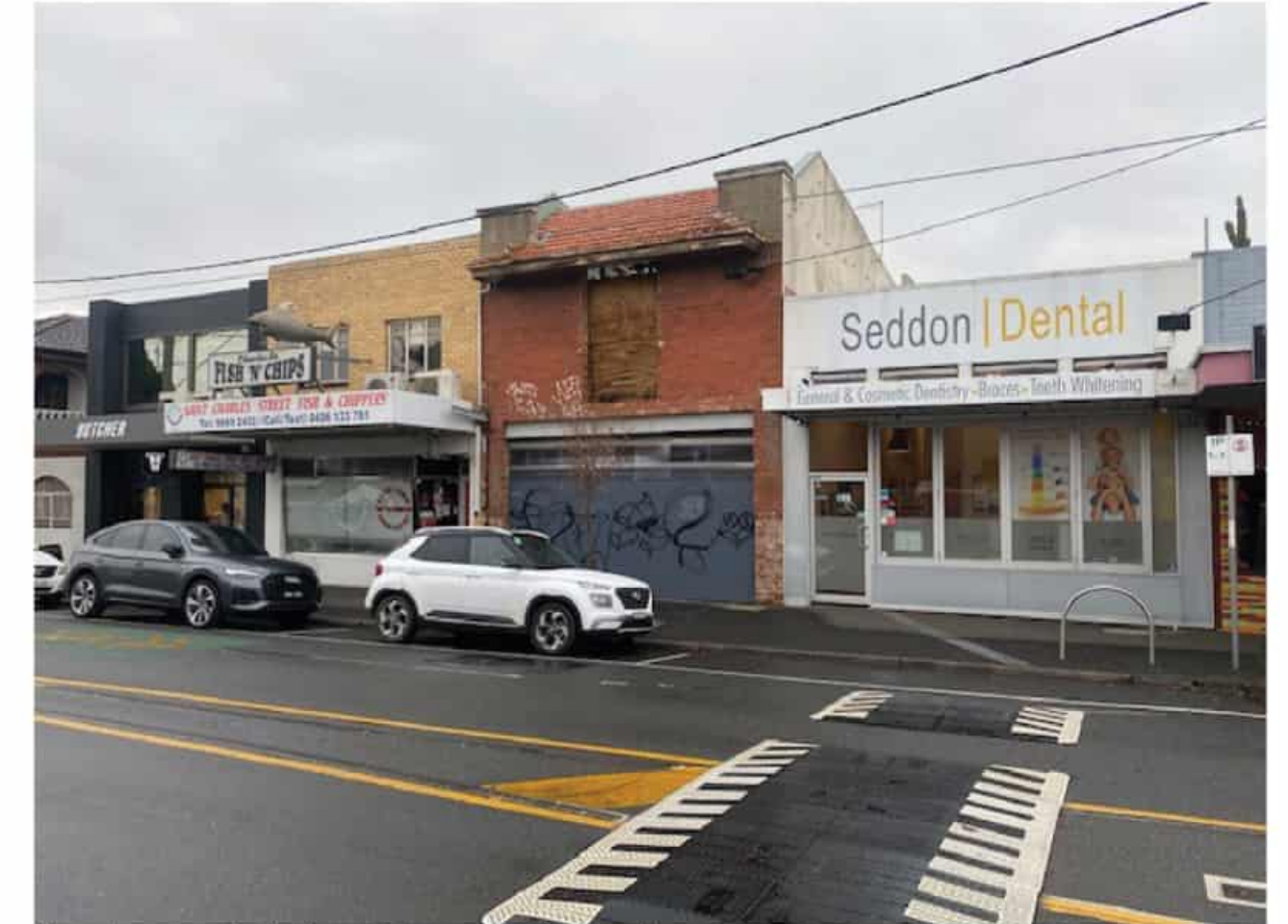
Long term neglected property on Charles Street
